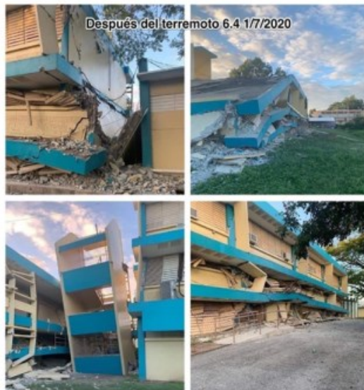
Agripina Seda School in Guánica After 6.4 earthquake Jan 7, 2019
