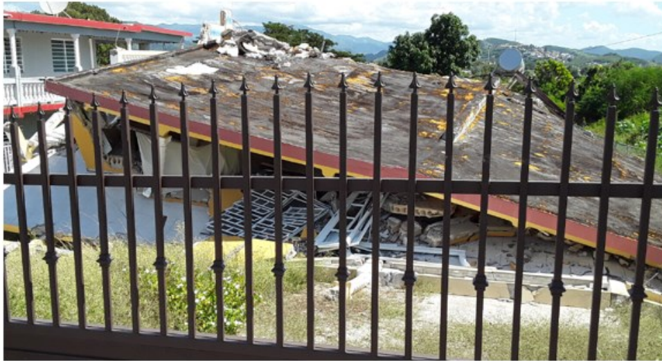
Earthquake destroyed home, Yauco, Puerto Rico, January 2020
